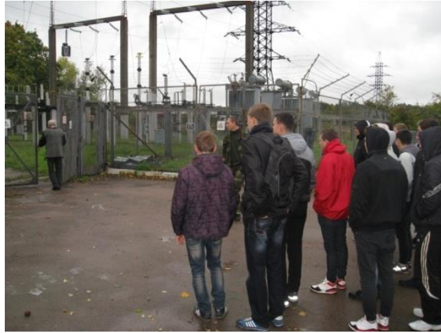
Figure 1. The beginning of the tour at the transformer substation 110/35/10 kV
